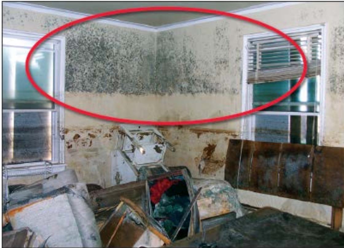
Figure 8-10. Typical interior flood damage to residential building in New Orleans, showing extensive mold growth (circle)
